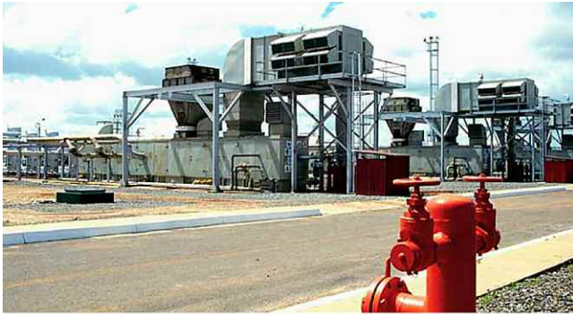
Figure 2. Air Inlet System with Filter and Silencer for a Gas Turbine Installation.
